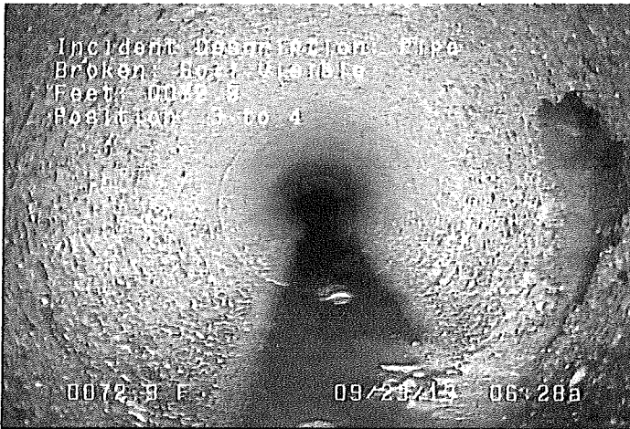
BSV - Pipe Broken: Soil Visible @ 72.9 ft.
