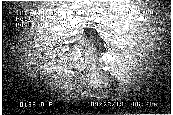
B - Pipe Broken @ 163.0 ft.
