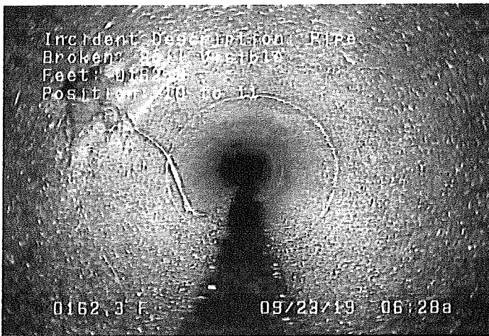
BSV - Pipe Broken: Soil Visible @ 162.3 ft.
