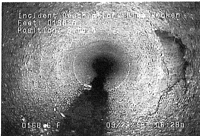
B - Pipe Broken @ 168.6 ft.
