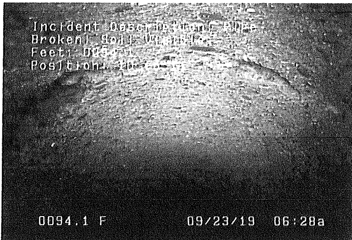
BSV - Pipe Broken: Soil Visible @ 94.1 ft.
