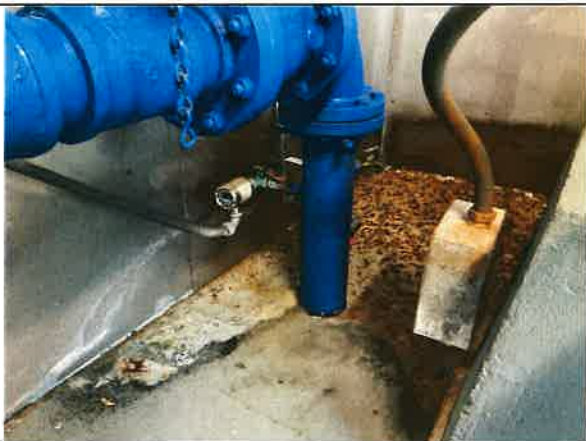
Picture One Notes: Location of said leak
